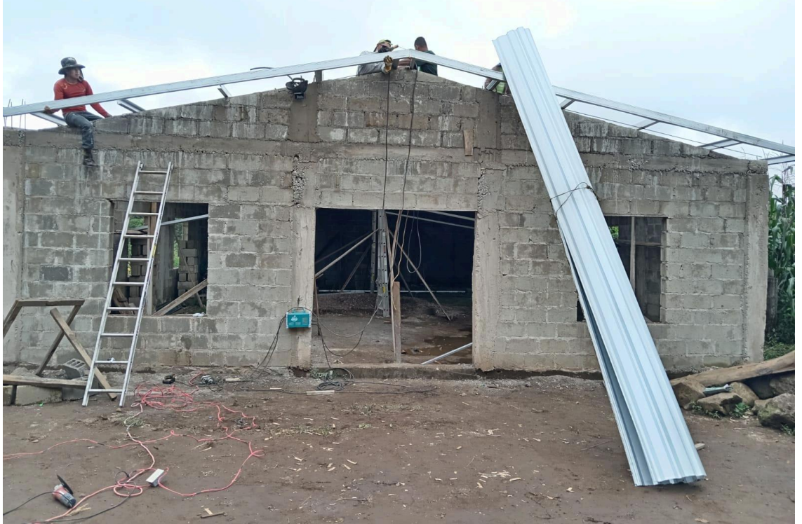
Progress in the Lenca Church plant construction in Quesuntega, Honduras. I plan to be there on November 15.
